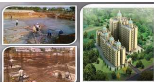
Project Location:- Bogadi Road, Mysore Project Description:- The structure was designed for 2B+G+9+Terrace Floors & execution is in progress. Project size & scale:- 63,000sqft & 6,50,00,000
