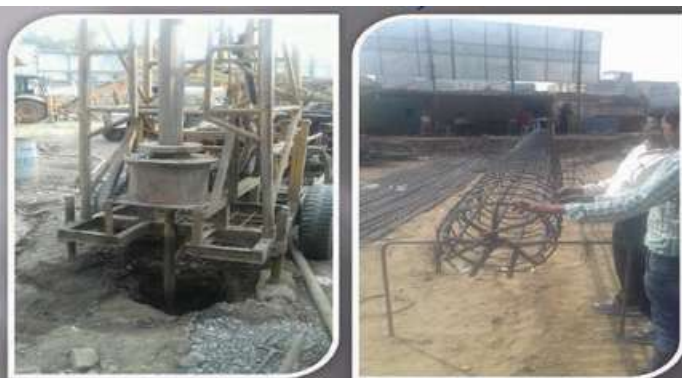
Project Location:- Surat Project Description:- Piling work for High rise Building in Surat.
