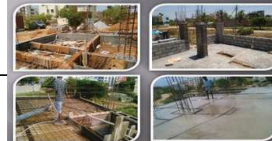
Project Location:- Kudlu Gate, Bangalore Project Description:- The structure was designed for G+2+Terrace Floors. Project size & scale:- 30'x40' & 60,00,000
