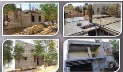
Project Location:- Sarjapura Road, Bangalore Project Description:- The structure was designed for G+2+Terrace Floors only & executed for G+1+Terrace Project size & scale:- 40'x70' & 84,52,000.
