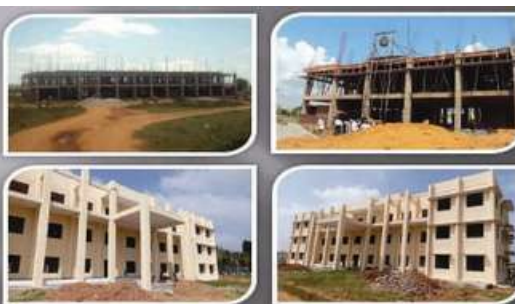
Project Location:- Jaynagar East, Tumkur Project Description:- 10,000 Sft Commercial Sales Tax Office
