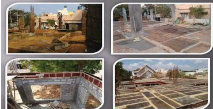
Project Location:- Sarjapura Road, Bangalore Project Description:- The structure was designed for G+2+Terrace Floors only & executed for G+1+Terrace Project size & scale:- 40'x70' & 84,52,000.
