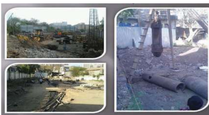
Project Location:- Surat Project Description:- Piling work for High rise Building in Surat.
